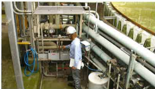
排水処理設備点検 Inspections of waste water treatment system 排水处理设备的点检
